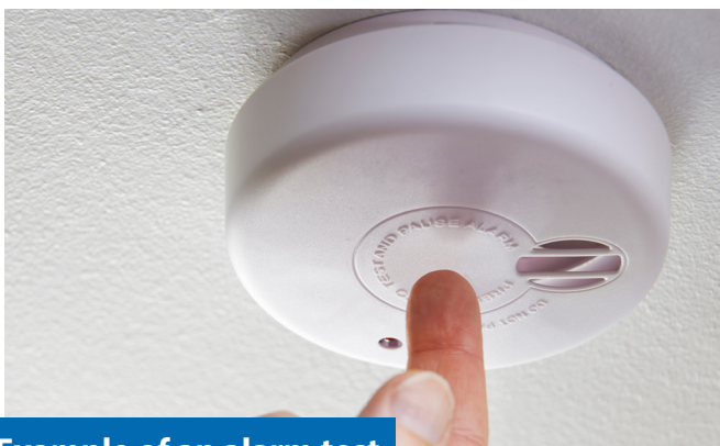
Example of an alarm test
